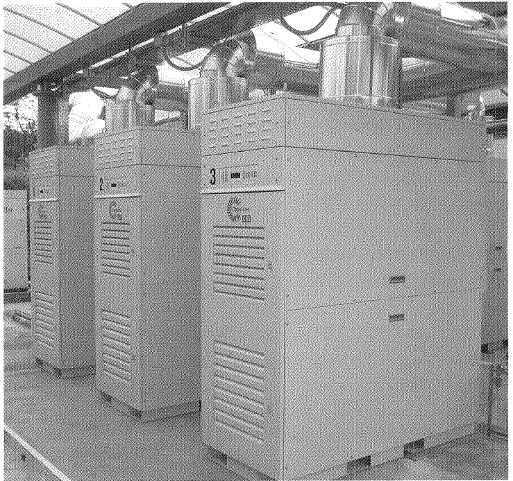
This CEM Ambiente landfill in Milan is the first in Italy to showcase Capstone microturbines.
