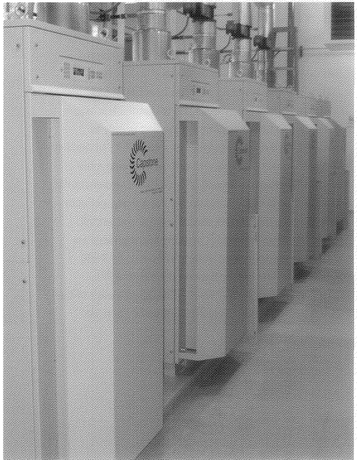
Twelve Capstone C65 Hybrid UPS microturbines are installed in Syracuse University's Green Data Center.
