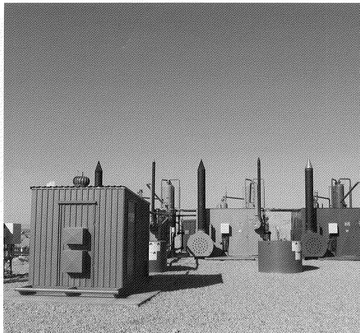
The remote Jonah Field wellsite uses a Capstone C30 microturbine to generate electricity to run the site's pumps.
