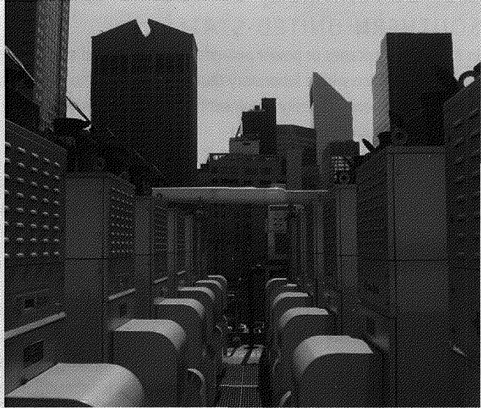
Twelve Capstone microturbines provide electricity and heat for this 35-story office tower in Manhattan.
