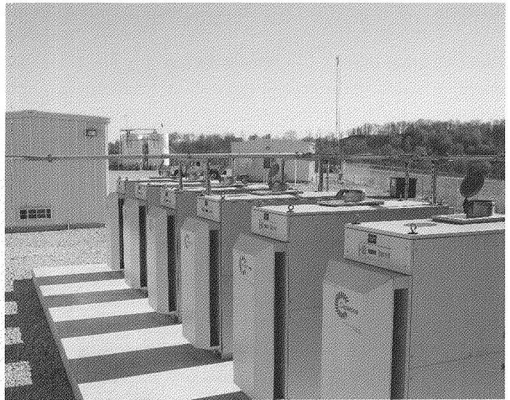
Capstone microturbines, operating in the Eagle Ford and Marcellus shale plays, generate reliable and clean power.
